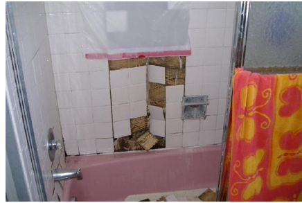
Figure 5. Total collapse of the shower wall.
