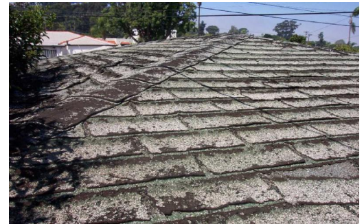
Figure 1. Premature roof deterioration resulting from lack of attic ventilation.
