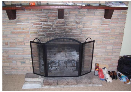
Figure 2. Soot above the fireplace can also indicate dangerous gases accumulating inside the home.
