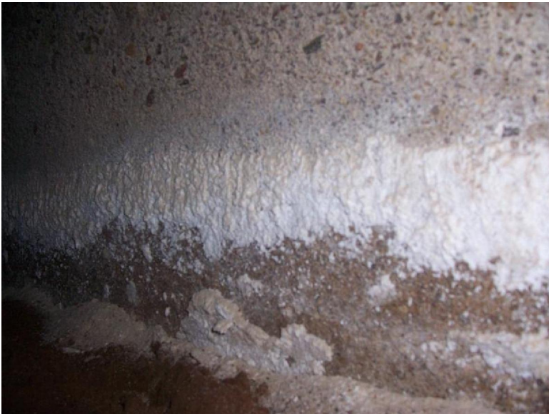
Figure 1. Excessive efflorescence on foundation wall.
